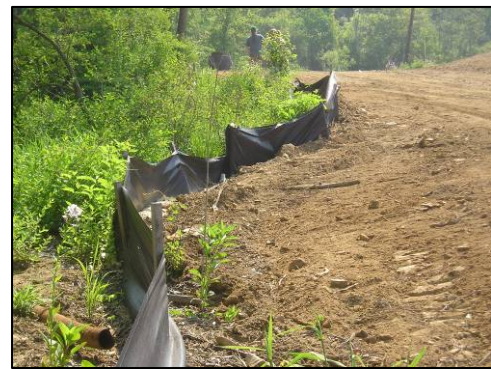
Siltation fences, as depicted in the photo, are a best management practice used to contain loose soil at construction sites
