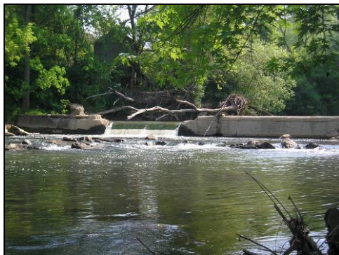
Breached dam on Connoquenessing Creek
