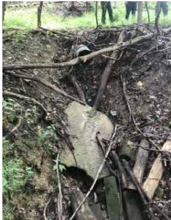
Severe Erosion from the Outfall Pipe from the Cedar Grove Lot
